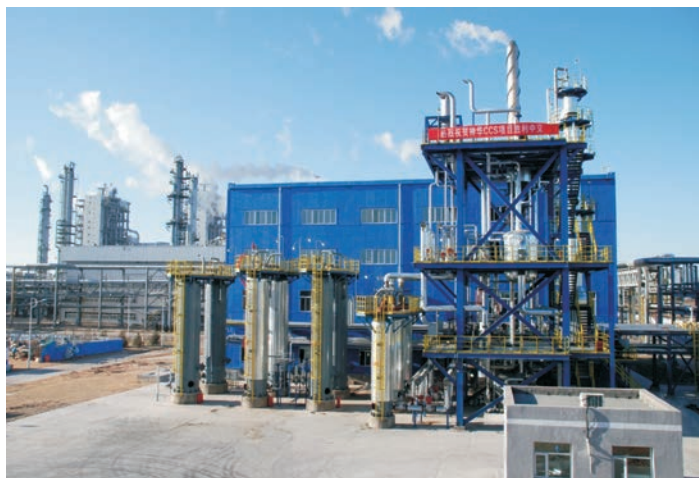
Shenhua Coal-to-Liquid CCS Project CO 2 Capture Plant
