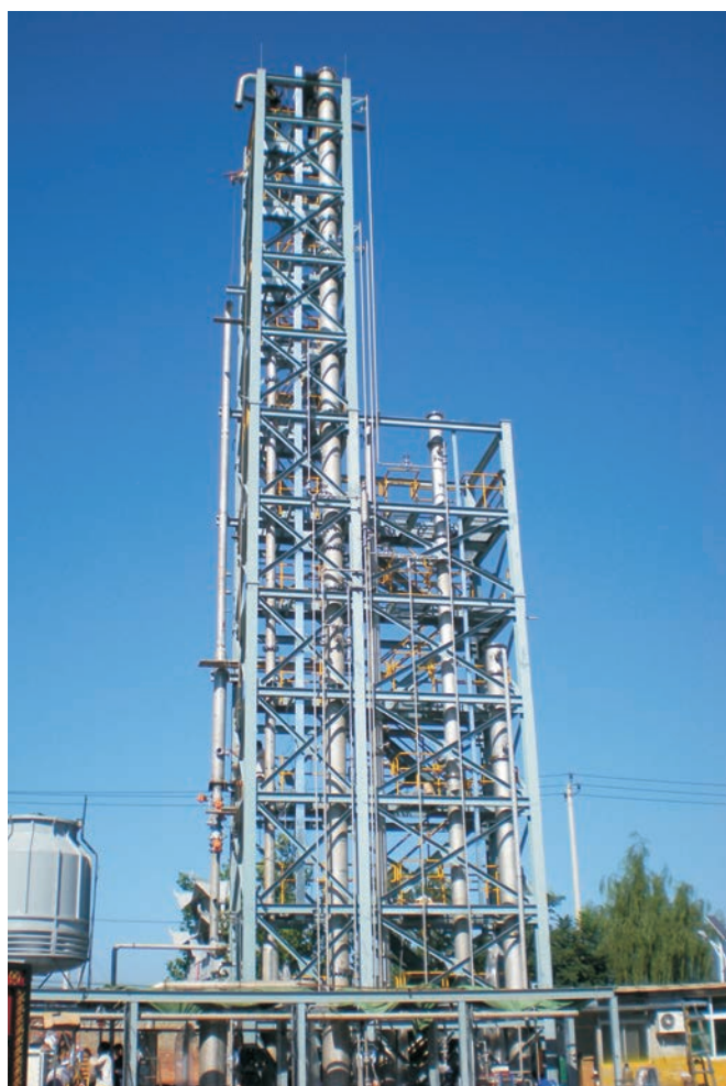
Beijing Pilot CO 2 Capture Unit from Simulate CCGT Flue Gas
